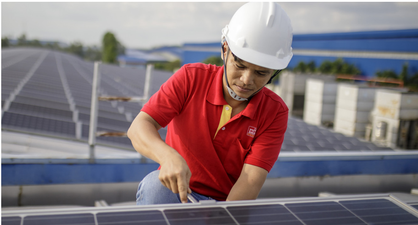
Solar Plant Sao Mai Corporation Vietnam © GIZ / Thomas Imo
